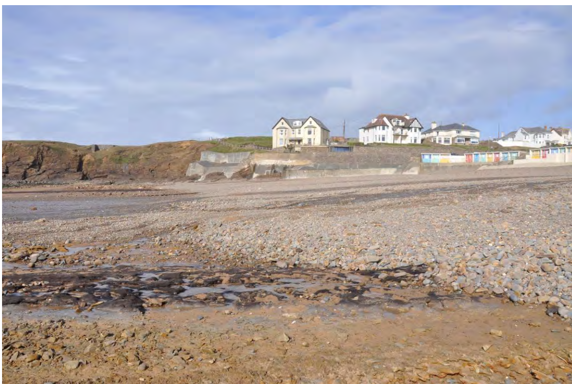
Figure 16: The relationship of the peat exposures to the modern shoreline which is protected by concrete revetments.
